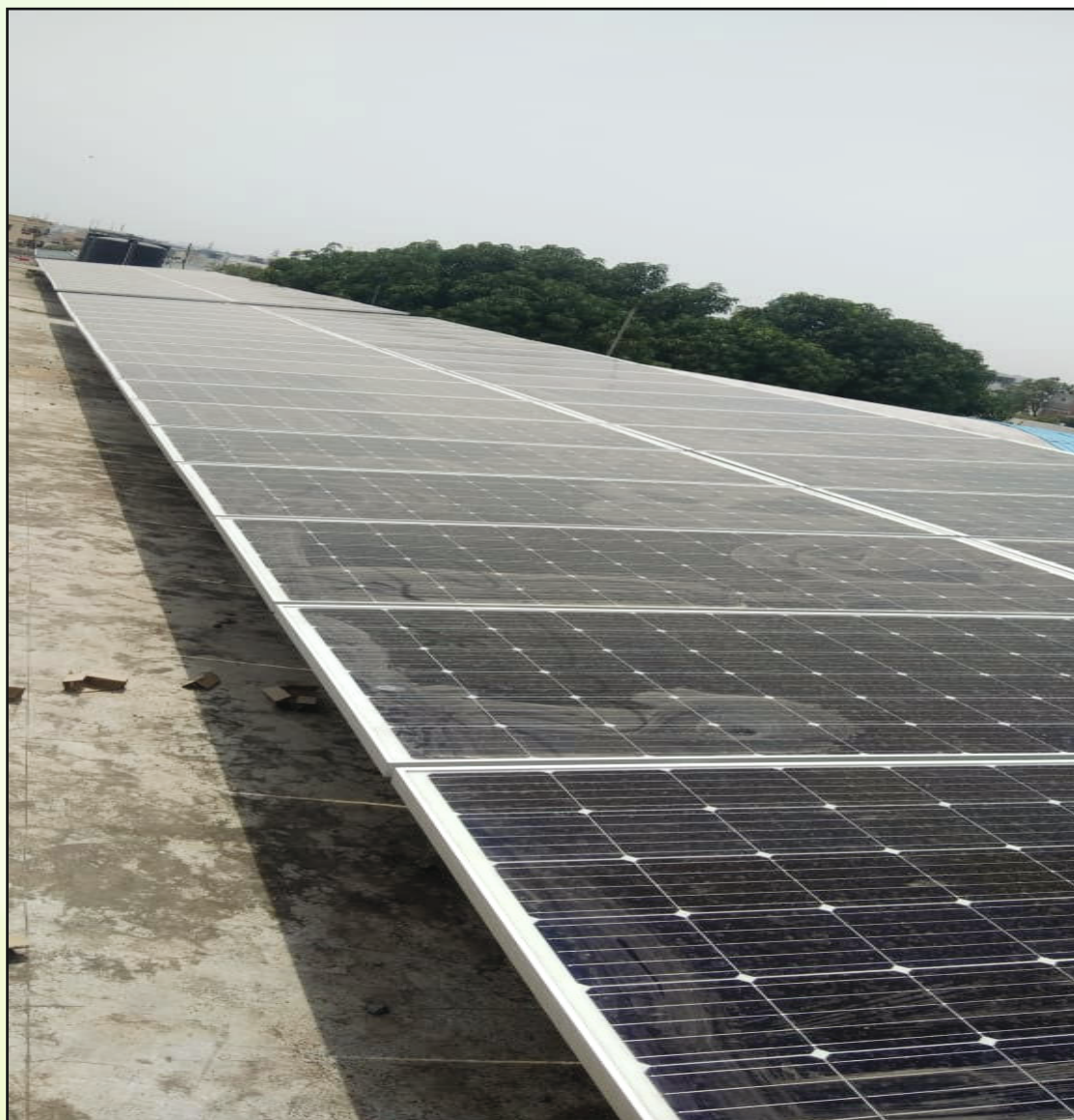
100 Kwp Solar Power Plant
